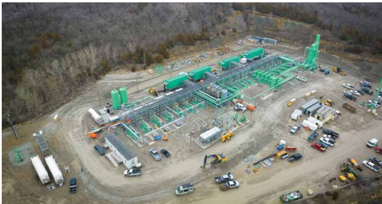
The Archaea Modular Design allows plants to be built on skids with interchangeable components for faster builds. The plant is located in Shawnee, Kansas, just outside of Kansas City.
